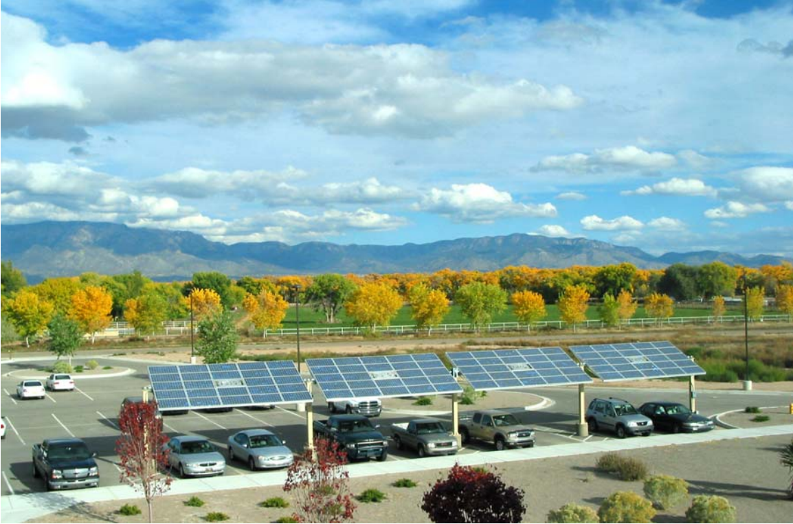
Visually integrated PV array and shade structure
